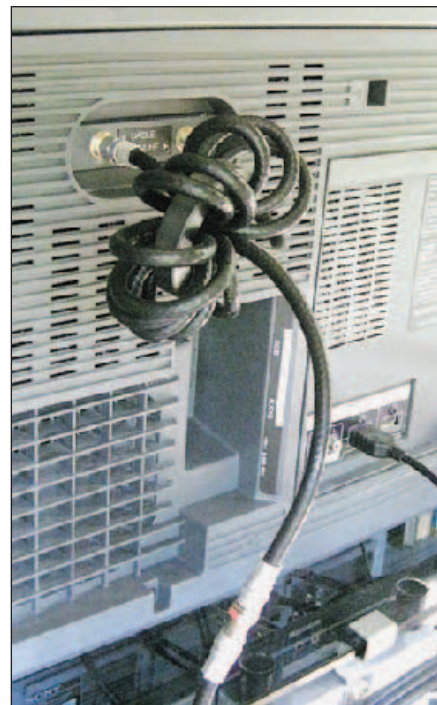
Figure 3 — The common mode choke installed on the coax input to the TV. This helped, but wasn't the final answer.
