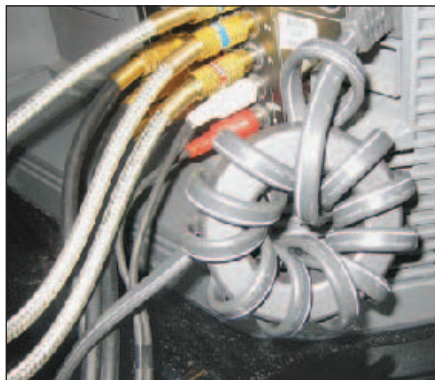
Figure 2 — A common mode choke on the power line, right at the receiver, attenuates RF on that path.
